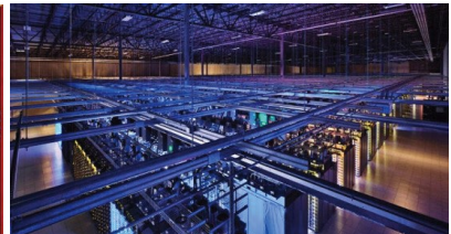
Data Center for Big Data Application
